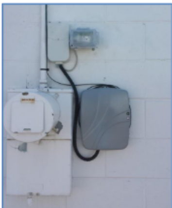
(Example of CPE installation)
